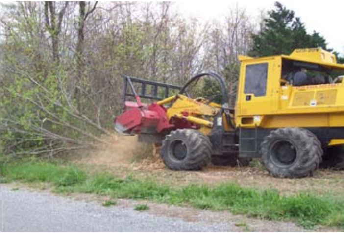
Carroll Electric's vegetation management crews clear right-of-ways, making way for its construction crews to come in and build utility lines.
